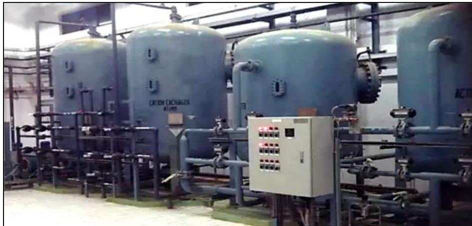
Fig.: Water DM Plant
